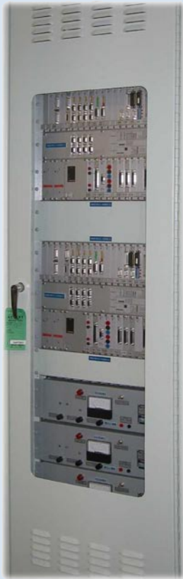
Fig. 2. One of the rugged Kontron PDCs for monitoring safety critical values in the CANDU reactor.
